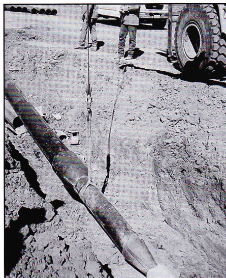
Figure 3. Bursting tool prior to pull-through. Note that the bursting head is at the bottom of the photograph, and that the pipe to be installed follows the bursting head. The pipe will be installed simultaneously with the pipe being burst into the surrounding soil. Photograph courtesy of TT Technologies, Inc.
